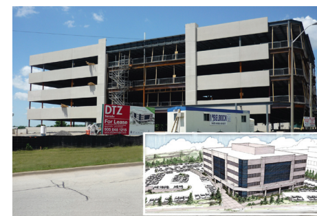
Construction of Takeda's new Mississauga location at 6750 Century Ave. Inset: Artist's rendering
